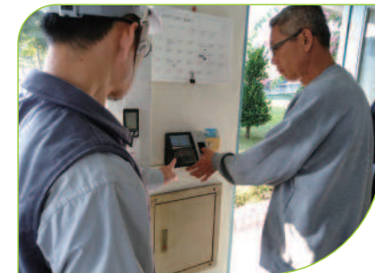
The facial and fingerprint recognition system was installed to control the entering contractors
