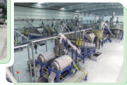
Working Line for PET Bottles Cleaning
