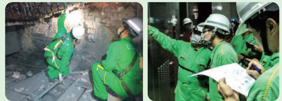
• ECOVE staff carries out preventive and corrective maintenance for equipment (left : stoker interior maintenance ; right : fire protection system inspection)
