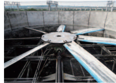
Cooling Tower Fan Units at Wurih Plant before Replacement
