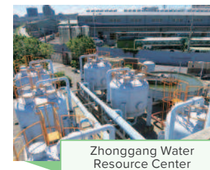
New Taipei City Gravel Water Treatment Plant
