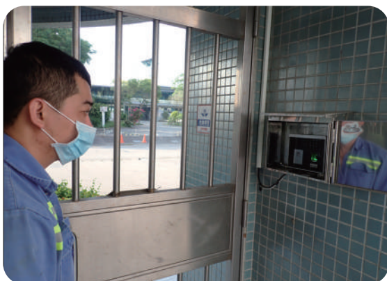
Installation of facial and fingerprint identification systems to facilitate the control of contractors' entry qualification
