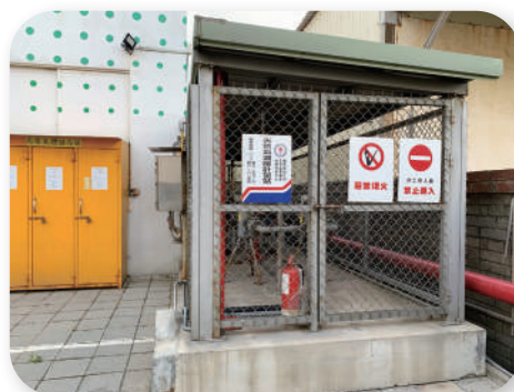
Replacement of heavy oil with natural gas.
