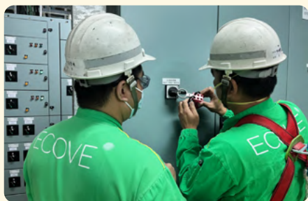
Equipment isolation tag
